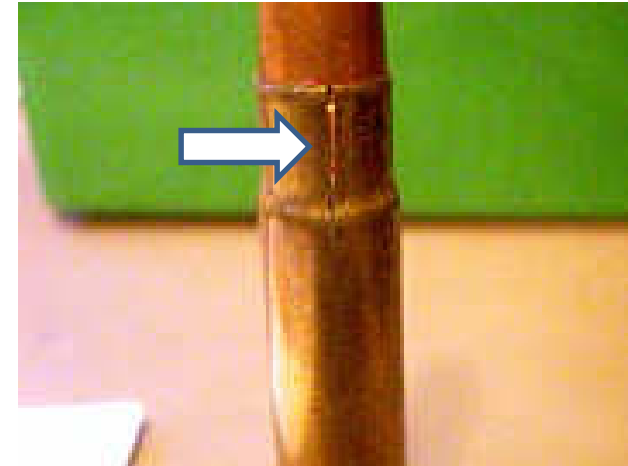
Fig.18. Classic example of season cracking http://en.wikipedia.org/wiki/Season_cracking
