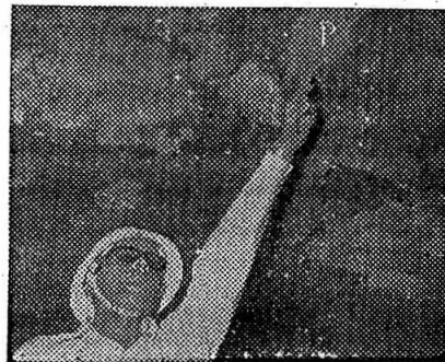
Fig. 4 Plastic patches in the roof of Rail Mill, reheating furnace No. 2 in the soaking zone (after a year of service)
