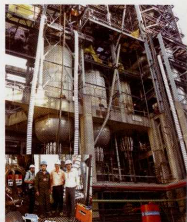
Fig- 6: Catalytic reactor unit of oil Industry where NML team carried out structural health monitoring using GMI based sensing device
