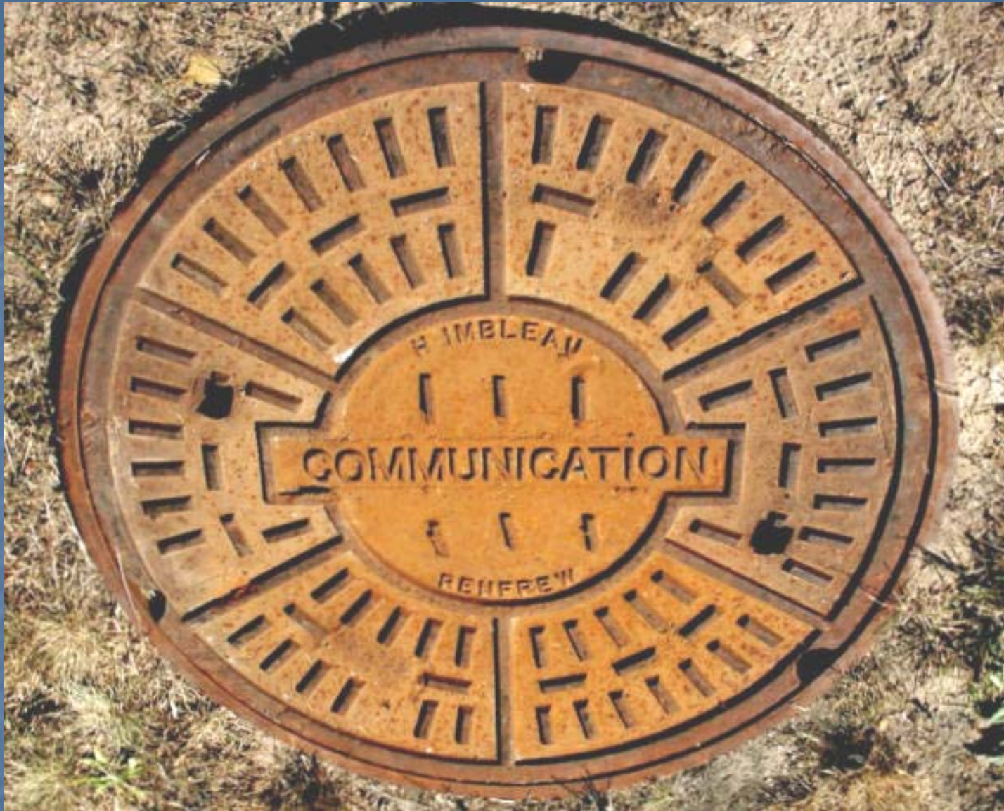
Active Corrosion on Carbon Steel Manhole
