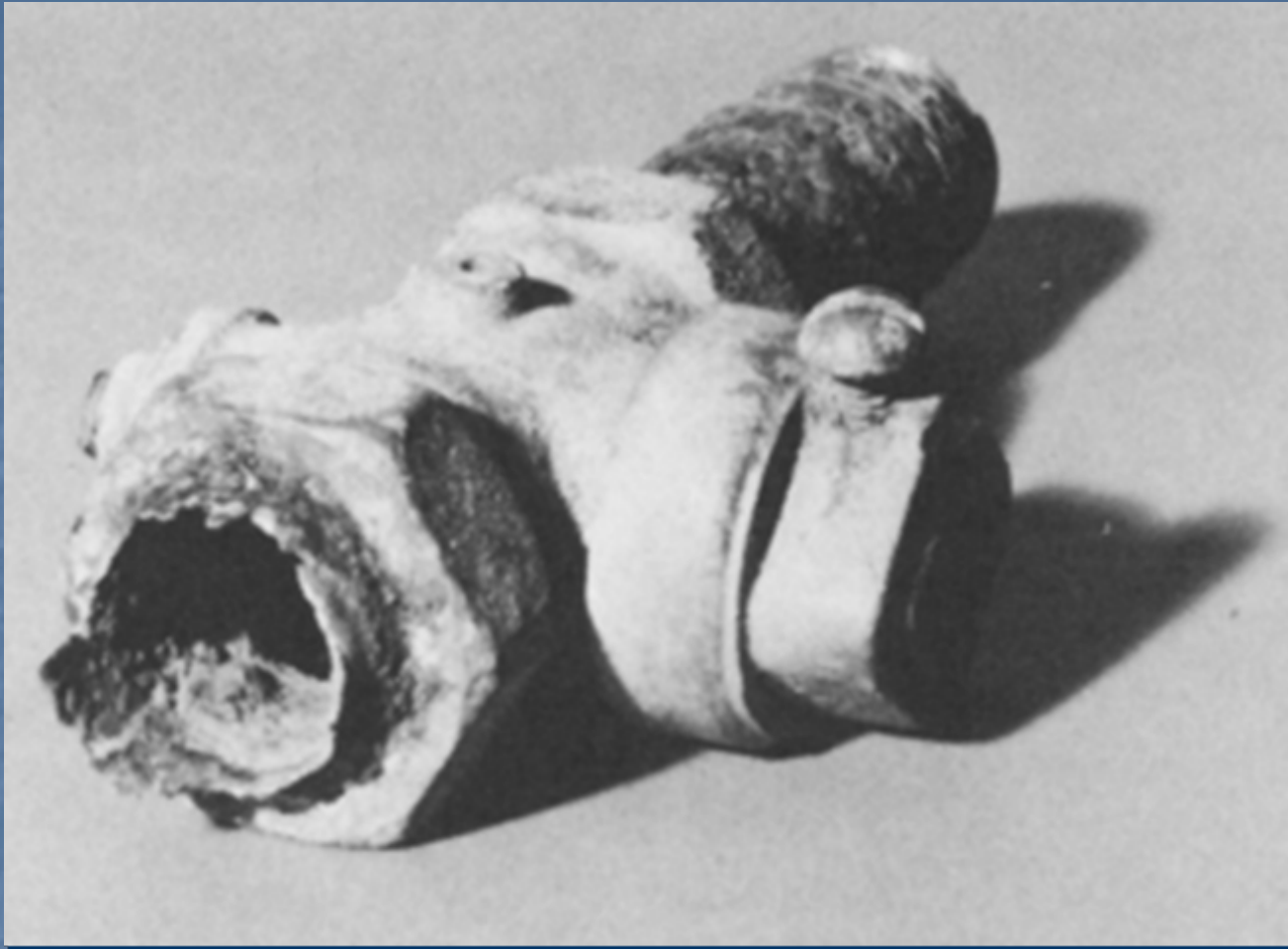
Galvanic corrosion of steel pipe at brass fitting in humid marine atmosphere
