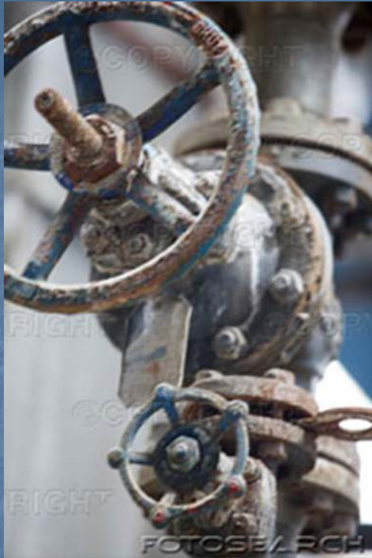
Pressure Valve in Petrochemical Plant
