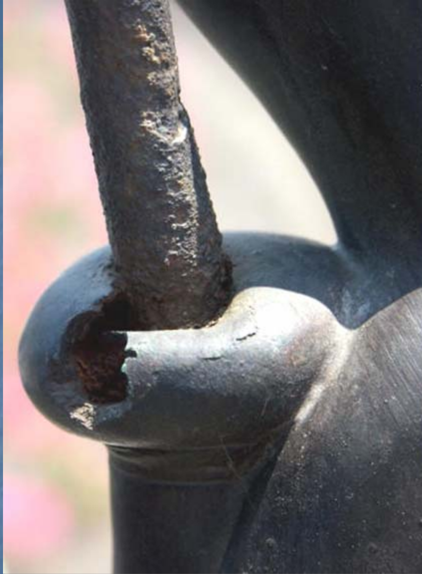
Stress Corrosion Cracking in a bronze component
