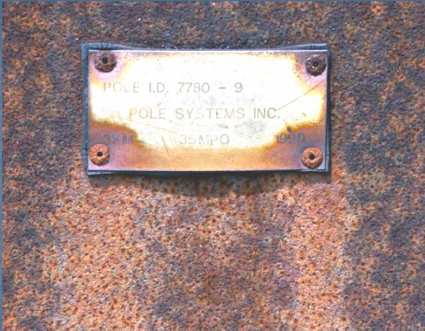
Galvanic Corrosion Couple between Steel and Brass
