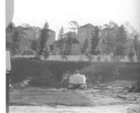
HARD HATS REQUIRED: The construction workers surveying what will eventually become the Engineering Parking Structure. Construction began in September 2004.
