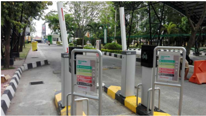
Fig.9. E-Gate system for the in lanes at main entrance
