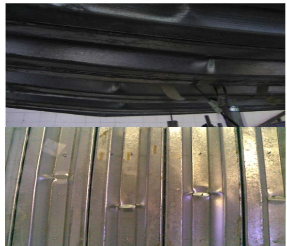
Fig. 4 Failure due to local buckling
