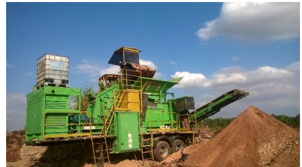
Figure 20. Mobile C&DW recycling facility located in São Paulo State.
