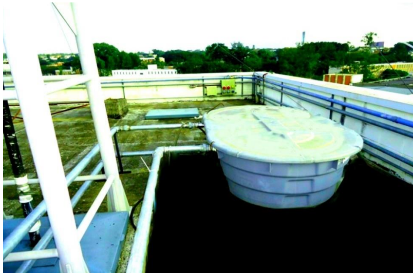
Figure 3. 6- Water main tank
