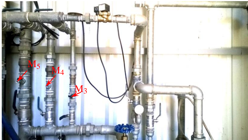
Figure 3. 7- Pressure transmitters M3, M4, M5
