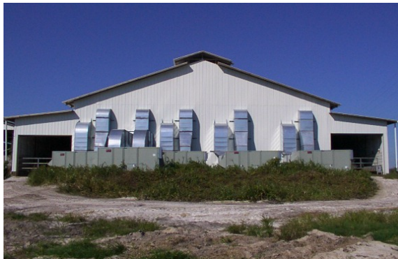
Figure 2. End of Barn B with air-conditioning equipment.
