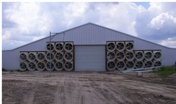
Figure 5. Exhaust fans on tunnel-ventilated barn (Barn C) with sprinkler evaporative cooling system.
