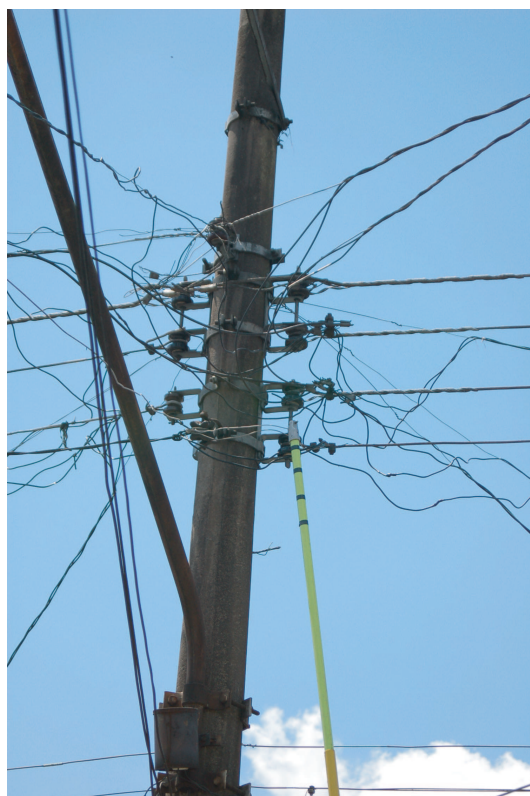
Fig. 4 Wiring of a typical pole connection in a poor region of the AES Eletropaulo concession area in the city of São Paulo.
