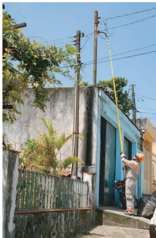
Fig. 3 A linesman installing the electronics device in a wiring connection of AES Eletropaulo.
