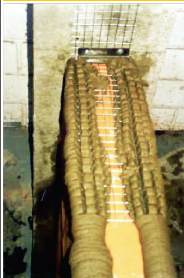
Figure 3 – Photo of an masonry/column Joint with an electrowelded metallic mesh fixed to the column using angles and metallic pins (7)
