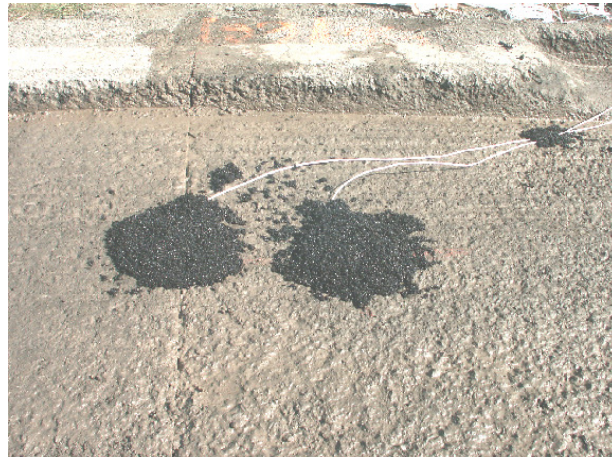
Figure 15.- Cracked and continuum asphalt layer
