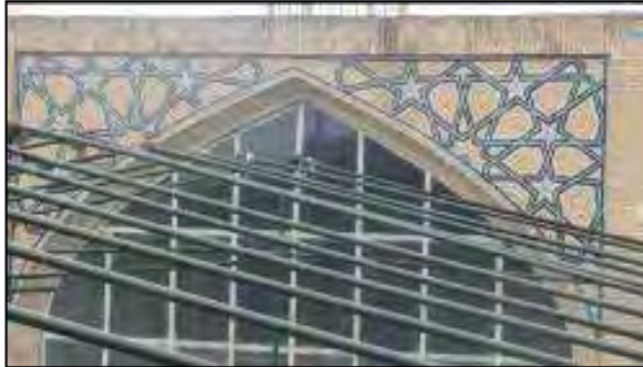
Figure 11. A gere accomplished in the southern-side spandrel
