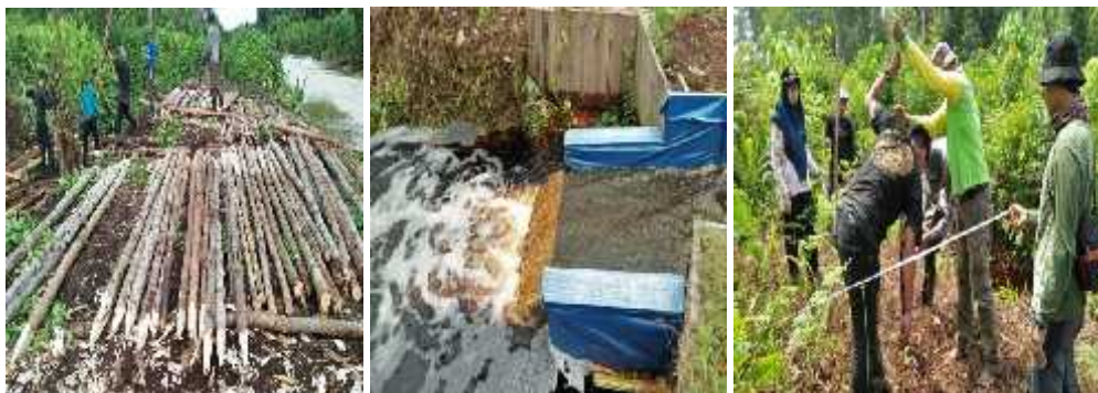
Picture 1: The Building of The Stuck Canal and The Monitor Well by Involving the Society Group of Lukun Village
