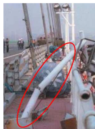
Fig 1. Cable damage in Haiyin Bridge [4].
