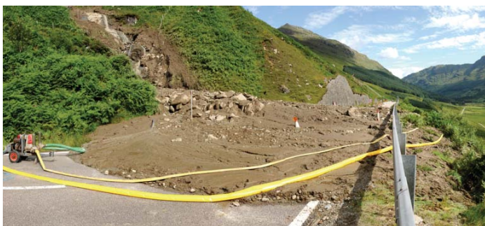
Landslide debris blocking the A83, Rest and Be Thankful, August 2012. Image © NERC
