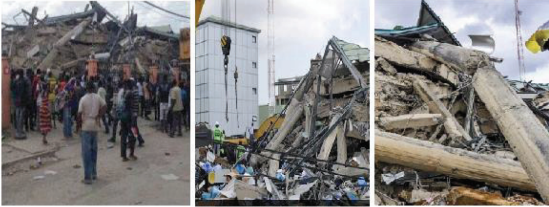
External View of Building after Collapse
