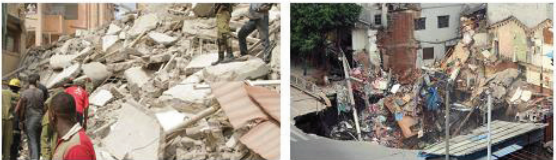
External View of Building after Collapse
