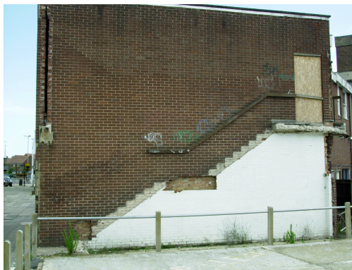
Figure 5. This is a photo of a building that has been partially demolished; this suggests a type of palimpsest, suggesting that there has been a memory to this site, a previous experience that has now been removed
