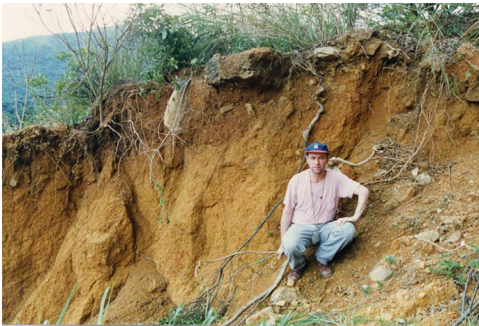
Plate 16 - Made Ground Exposed in the Main Scarp of Landslide Scar 2 (Plate Location Shown on Drawing EG503) (Taken on 7/8/97) GS 97/93C/14
