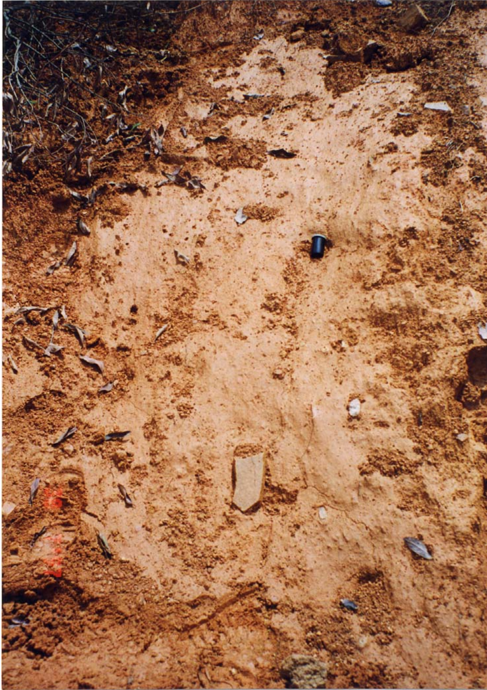
Plate 12 - Planar Slickensided Surface of Rupture Exposed below the Crown of Landslide Scar 1 (Plate Location Shown on Drawing EG503) (Taken on 30/7/97)
