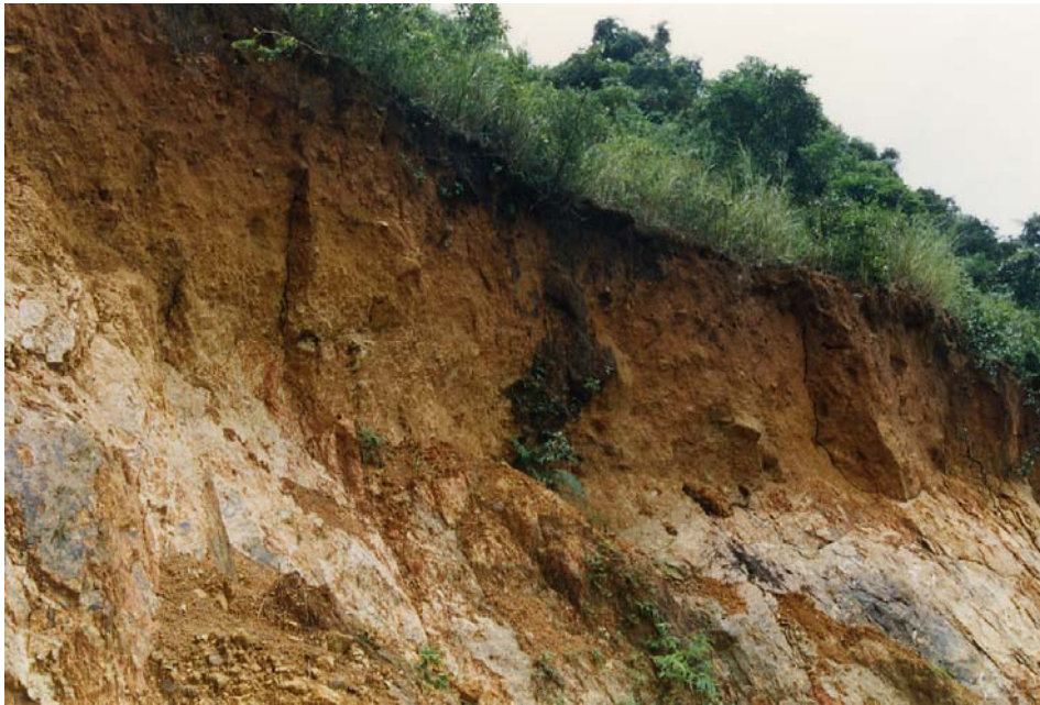
Plate 27(a) - Main Scarp of Landslide Scar 5 Viewed from the West - Note Older Mottled Colluvium, Dark Brown Staining on Scarp Surface and Sharp Interface Between Colluvium and Saprolite (Taken on 8/8/97) GS 97/107/33
