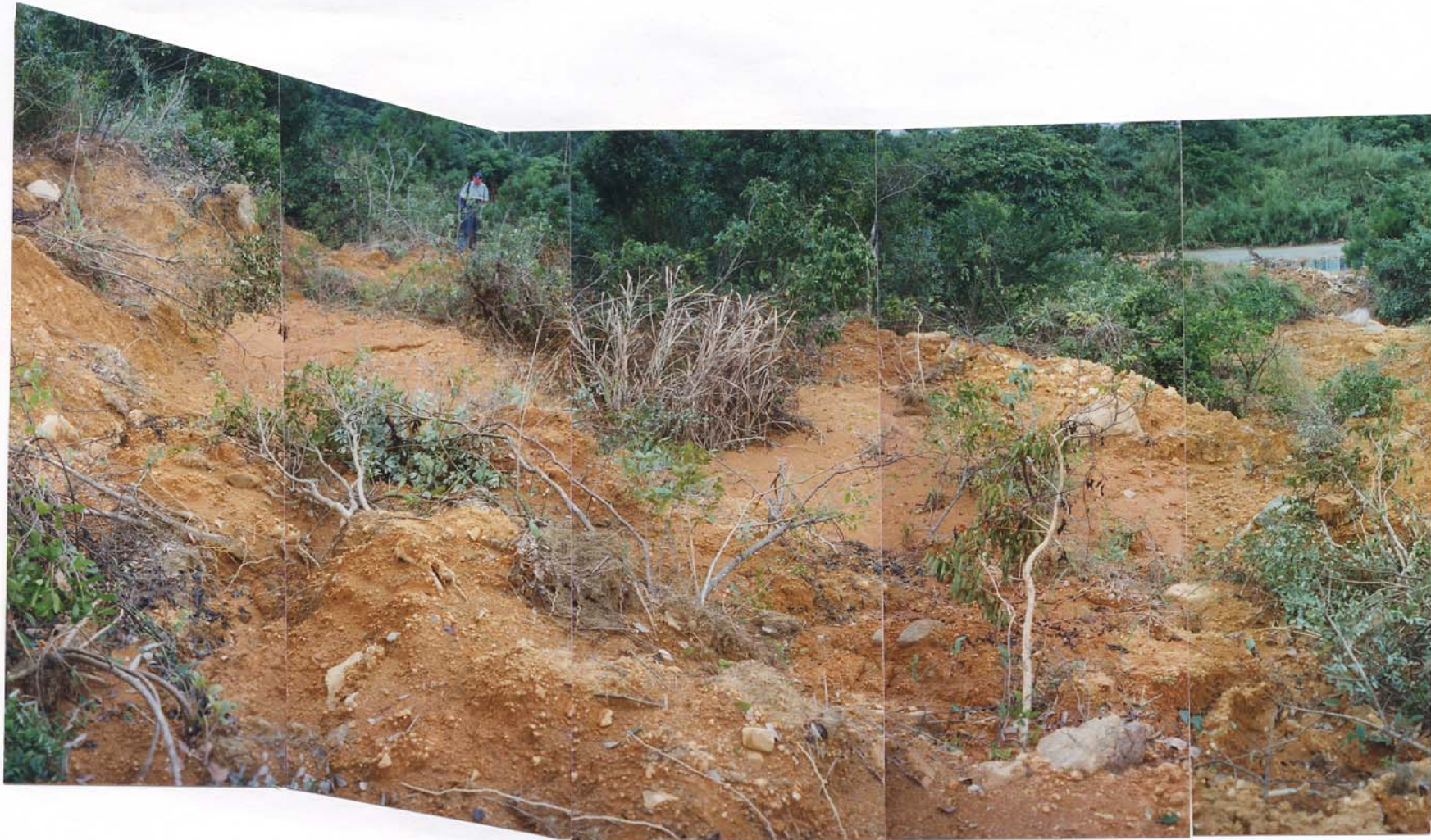
Plate 13 - Flat Area of Deposition and Debris Mound in Area Up-Slope of the Intact Debris Raft in Landslide Scar 1 (Plate Location Shown on Drawing EG503) (Taken on 30/7/97)
