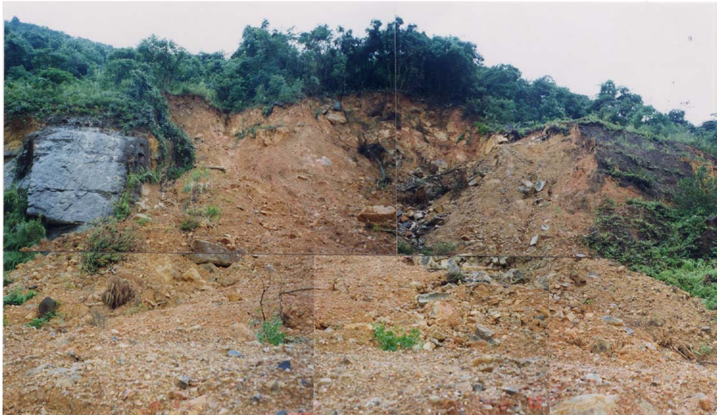
Plate 26 - View of Landslide Scar 5 from the South-East (Plate Location Shown on Drawing EG503) (Taken on 12/8/97)
