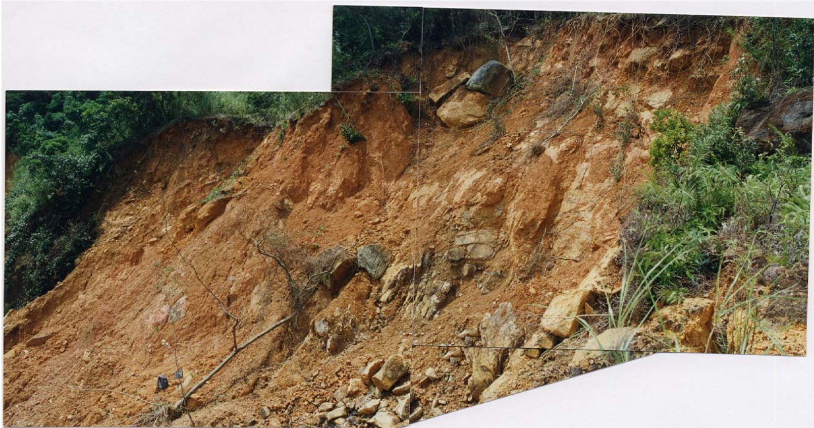
Plate 23 - Joint Controlled Surface of Rupture Exposed in Landslide Scar 4 (Plate Location Shown on Drawing EG503) (Taken on 6/8/97)
