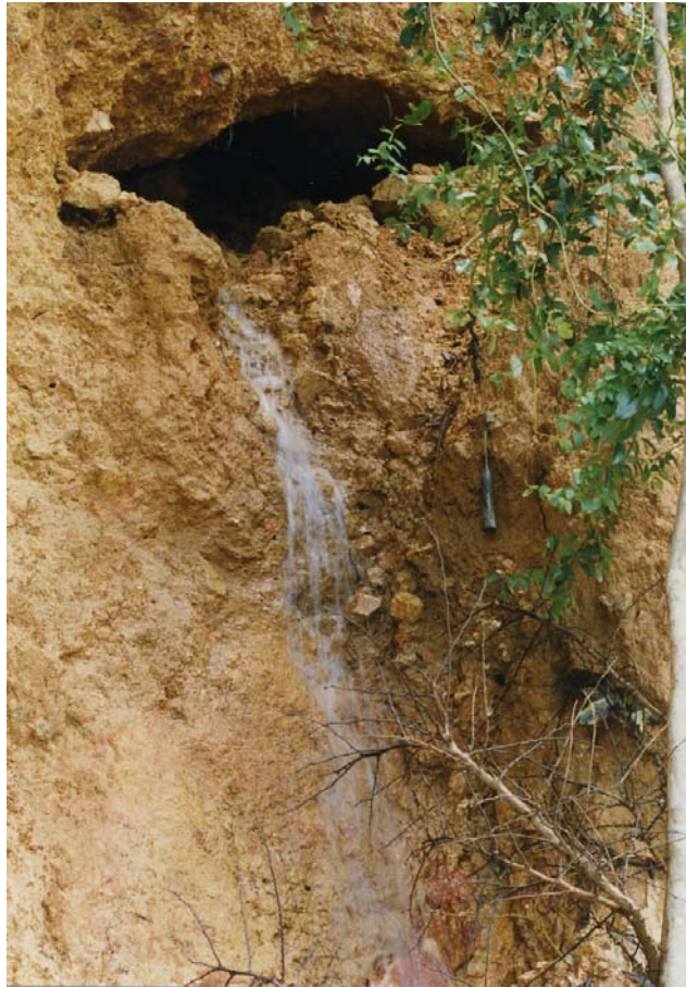
Plate 28(b) - Soil Pipe with Medium Flow (Plate Location Shown on Drawing EG503) (Taken on 8/8/97) GS 97/107C/30
