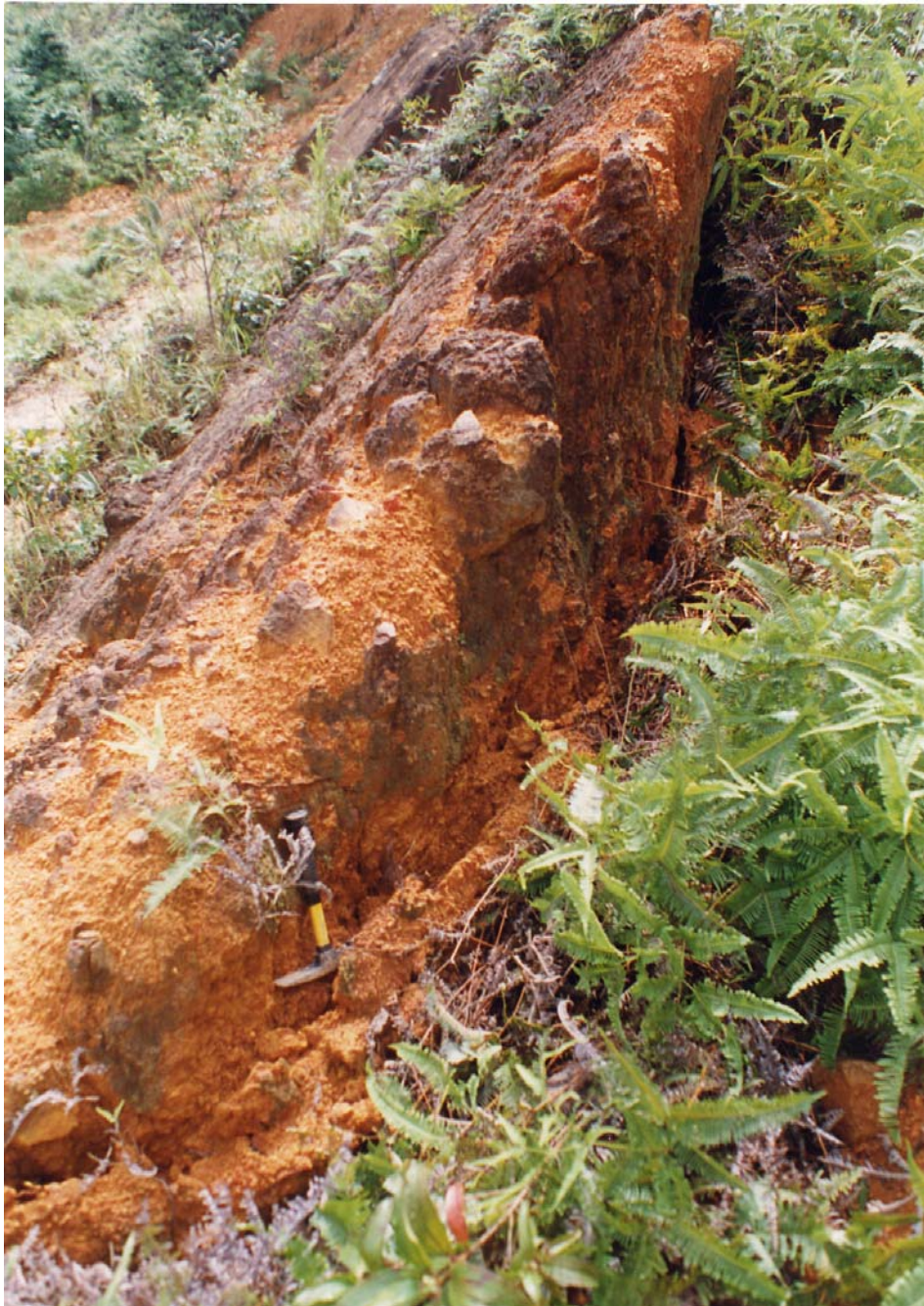
Plate 20 - Counter-Scarp Tension Cracks above Landslide Scar 3A Indicating Possible Toppling Mode of Failure (Plate Location Shown on Drawing EG503) (Taken on 10/7/97)
