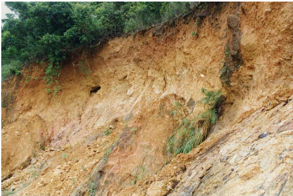
Plate 27(b) - Main Scarp of Landslide Scar 5 Viewed from the East - Note Large Soil Pipe (Plate Location Shown on Drawing EG503) (Taken on 7/7/97) GS 97/53/15
