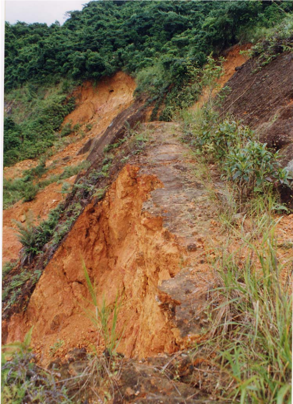
Plate 19 - Landslide Scar 3A Viewed from the South-East (Plate Location Shown on Drawing EG503) (Taken on 7/7/97)
