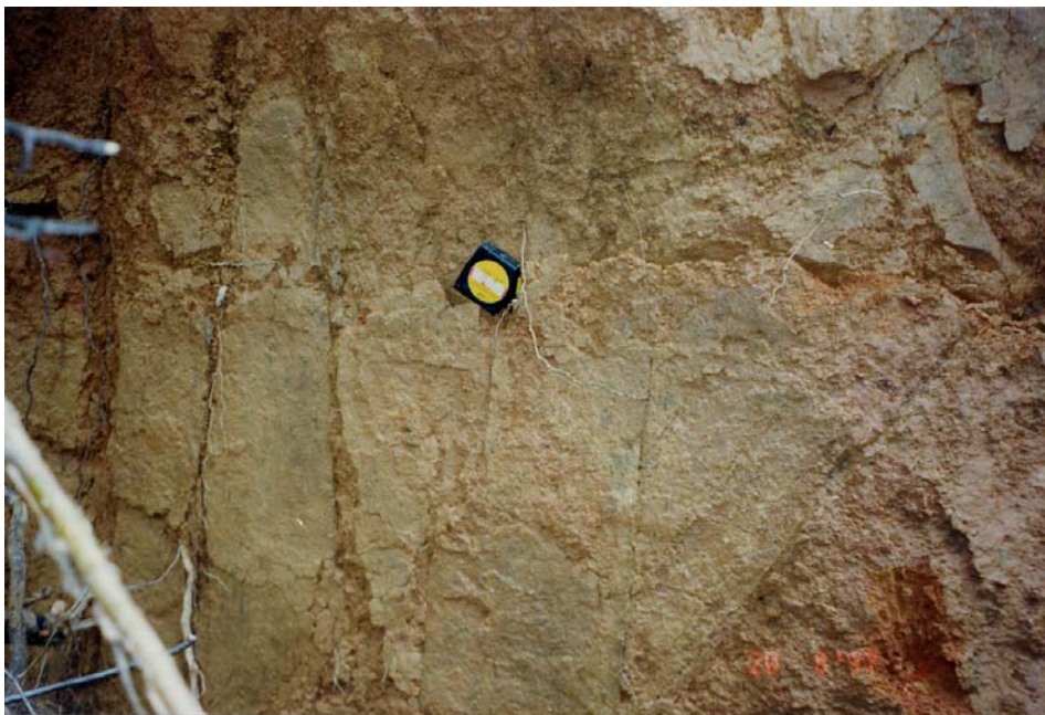
Plate 10 - Main Scarp Controlled by Relic Joints within Saprolite (Plate Location Shown on Drawing EG503) (Taken on 20/8/97)
