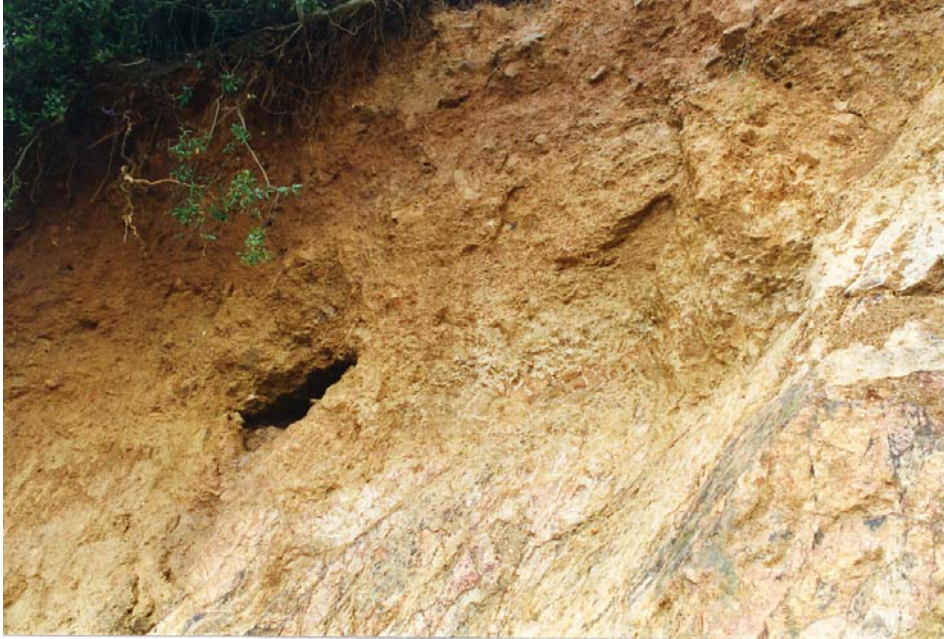
Plate 28(a) - A Large 1.5 m Wide Soil Pipe at the Old Colluvium-New Colluvium Interface Exposed in the Main Scarp of Landslide Scar 5 - Note Slight Seepage (Plate Location Shown on Drawing EG503) (Taken on 7/7/97) GS 97/53/07
