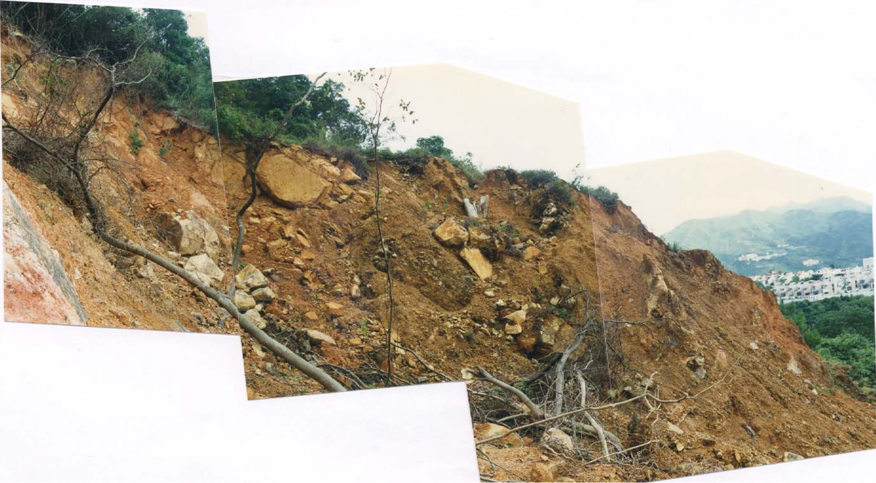
Plate 22 - Left Hand Flank of Landslide Scar 4 Showing Disrupted Rock Mass (Plate Location Shown on Drawing EG503) (Taken on 6/8/97)
