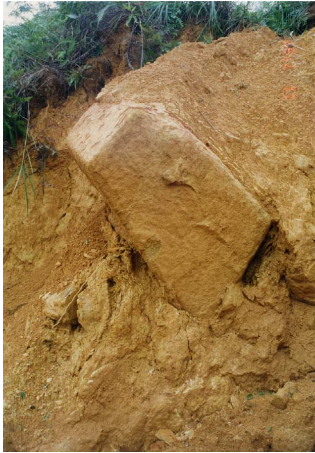
Plate 15 - Corestone Showing Evidence of Rotation Exposed in Right Hand Flank of Landslide Scar 2 (Plate Location Shown on Drawing EG503) (Taken on 10/7/97) EG 97/89/29
