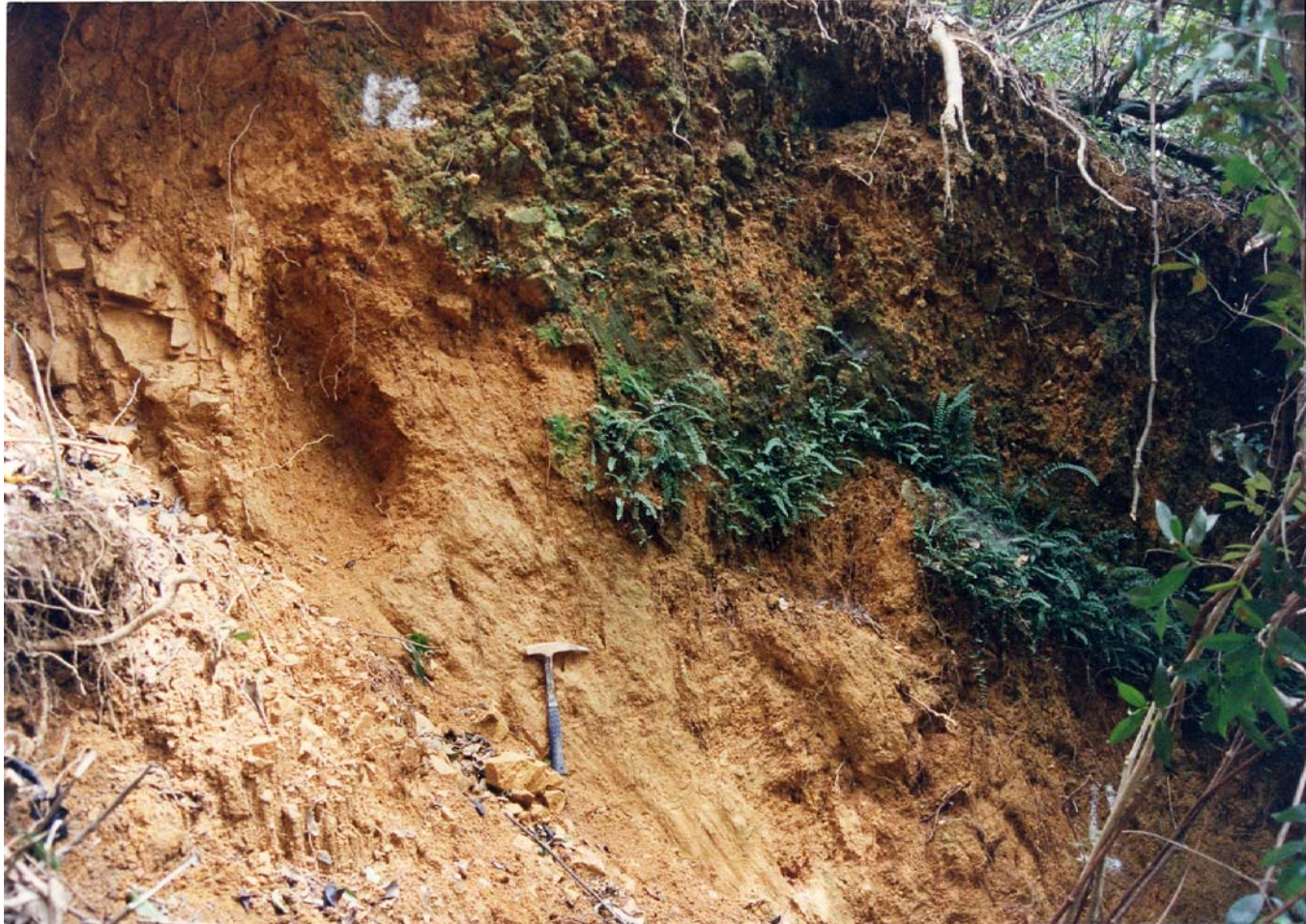
Plate 36(a) - Main Scarp Showing Vegetation Line Indicating at Least Two Phases of Movement Together with Old and Recent Slickensides on the Scarp Surface and a Rhyolite Dyke Contact (Plate Location Shown on Drawing EG503) (Taken on 26/9/97)
