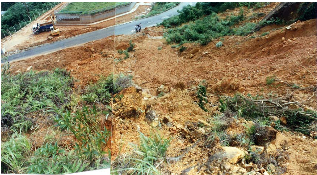
Plate 25 - Debrisflow-Earthflow Lobes from Landslide Scar 4A (Plate Location Shown on Drawing EG503) (Taken on 10/7/97) GS 97/64/10 - 11
