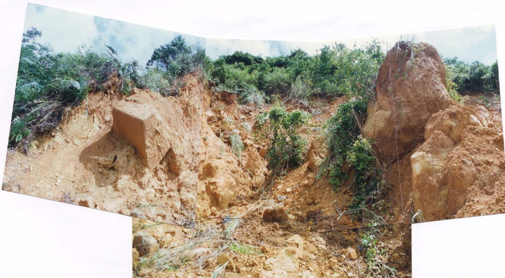
Plate 14 - View of Landslide Scar 2 Looking Up Towards the Main Scarp (Plate Location Shown on Drawing EG503) (Taken on 14/7/97)
