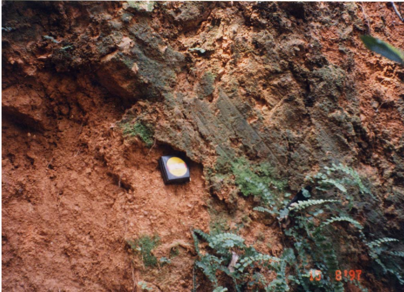
Plate 36(b) - Close-Up of Old Moss Covered Slickensides (Plate Location Shown on Drawing EG503) (Taken on 26/9/97)
