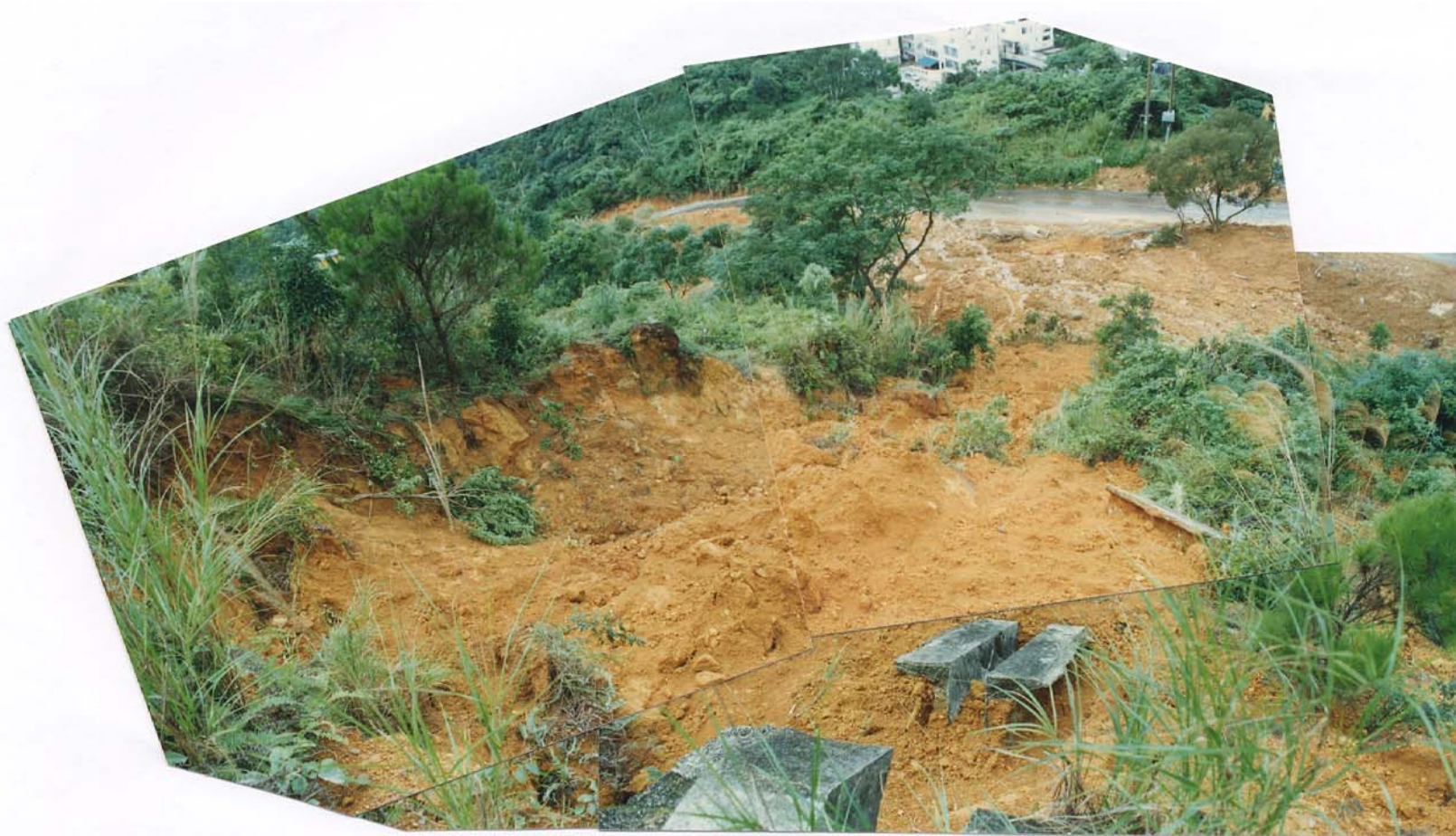
Plate 17 - View of Landslide Scar 3 Looking Down Towards the Left Hand Flank (Plate Location Shown on Drawing EG503) (Taken on 7/7/97)
