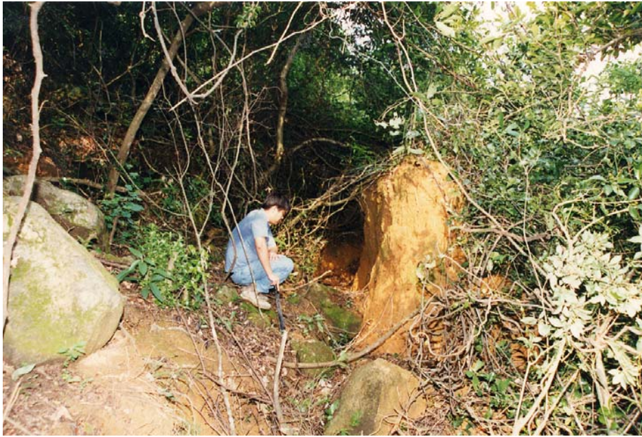
Plate 9 - Heaved Block of Saprolite or “Pop-Up Structure” within Main and Minor Scarp Complex (Plate Location Shown on Drawing EG503) (Taken on 3/9/97)
