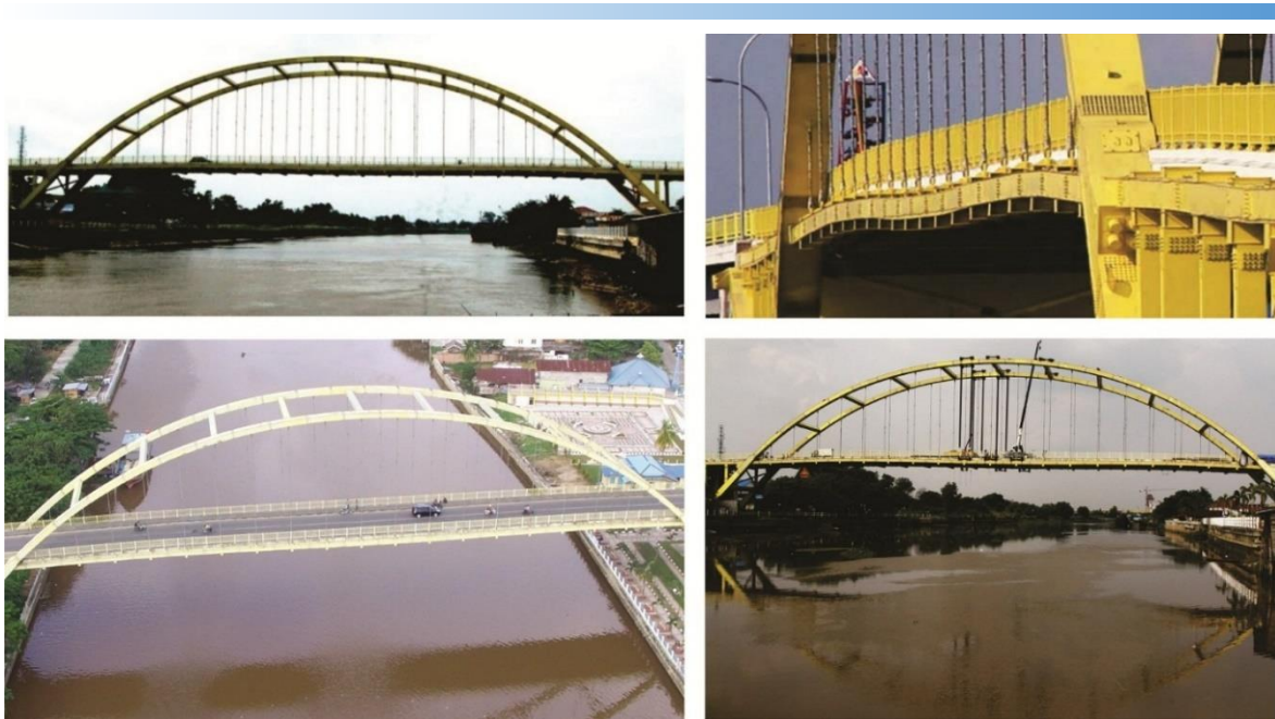
Fig. 7. Clockwise: Siak III bridge after being built completely; the deflection while used; repairing process; after repairing
