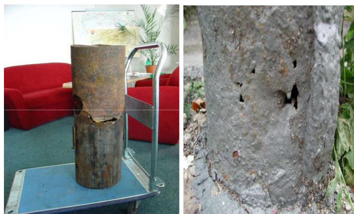
Fig. 1. Damaged lighting poles
