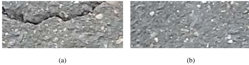
Figure 4. Example of dataset with (a) crack and (b) no crack
