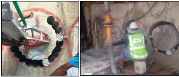
Figure 3 Stitch coring of secant bored pile to allow direct access of machine to ground [2]
