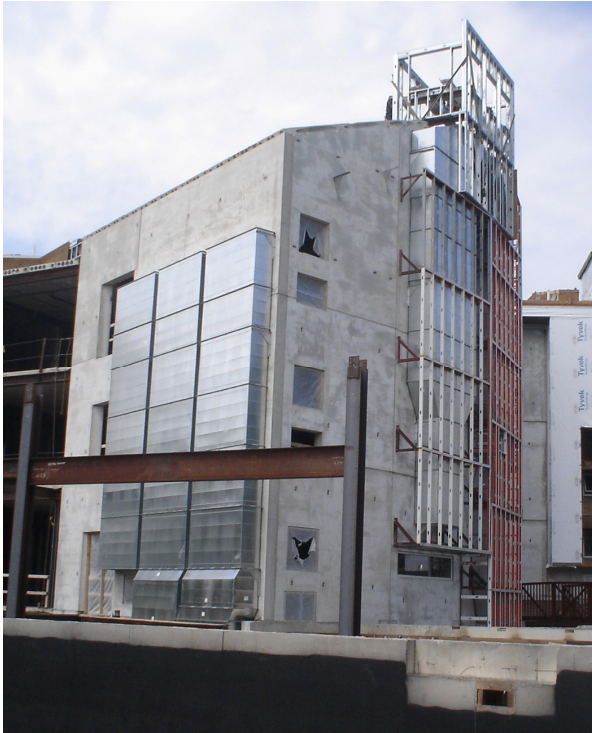
Figure 5: Pre-cast concrete structure with supply air ducts (left) and return air duct/stack (right), during rough framing. Source: (Author 2006)
