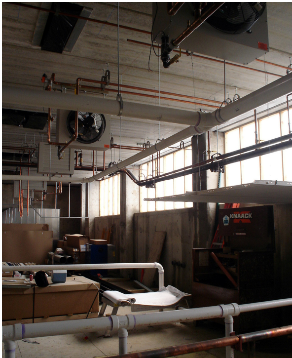
Figure 6: External fresh air intake supplies the lower level insulated ceiling plenum (air travels from right to left in this construction photo). Source: (Author 2006)
