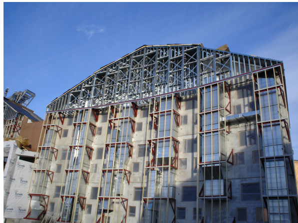
Figure 4: Pre-cast concrete structure with return air stacks during rough framing. Source: (Author 2006)
