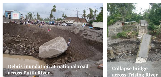
Figure 1. Damages due to debris flow disasters in the aftermath of 2010 Mt. Merapi eruption
