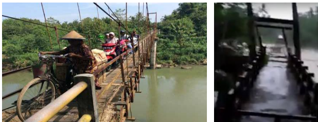
a). Nambangan Bridge (before and after the collapse)
