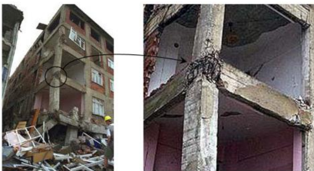
Figure 2. Joint panel damage caused by earthquake (Guner, 2016)
