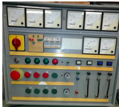
Figure 25: Controller of the inverter A.
