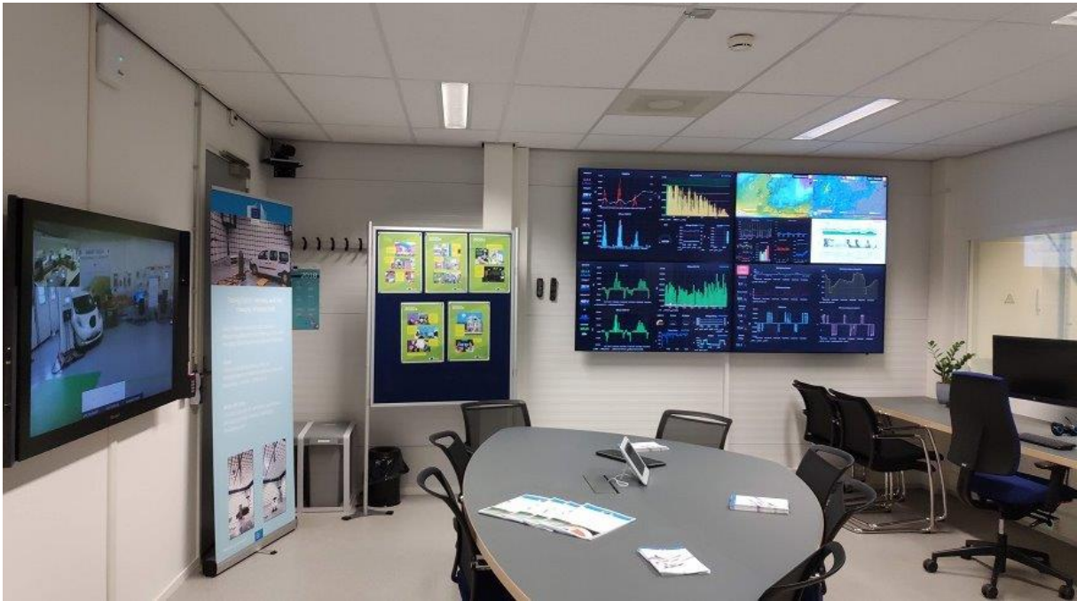
Figure 6. Control room SGIL, first floor
