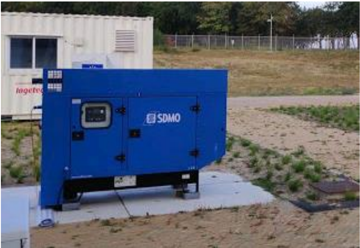
Figure 15. Diesel generator SGIL
