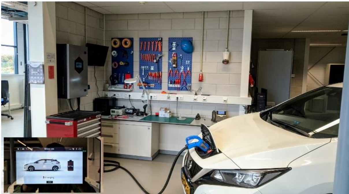
Figure 66. Vehicle to Grid (V2G) Charger, bidirectional flow of energy possible
