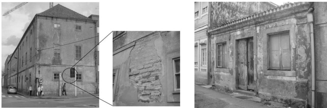
Figure 3.2.2 – Examples of degradation and abandonment buildings in Aveiro (Silva, 2011).
