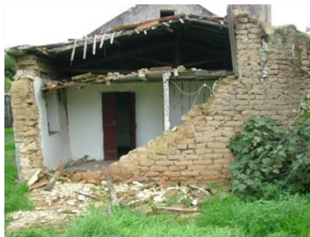
Figure 3.3.3 – Adobe house in Figueira da Foz, showing the materials degradation.
