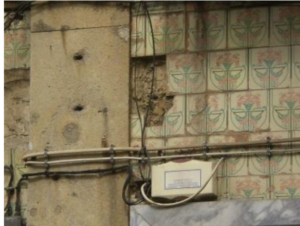
Figure 1 – Improper installation of services in old tiled facade
