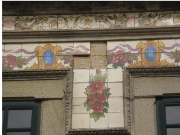
Figure 3 - Loss of the adhesive function of the mortars
