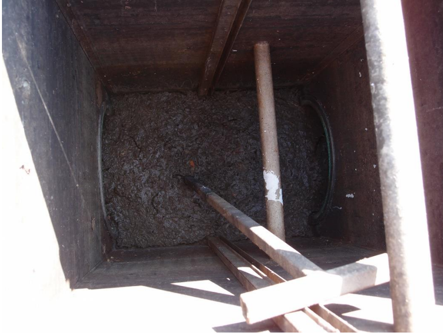
Figure 22. Water control structure that has become inoperable due to sedimentation on an easement in Calhoun County.
