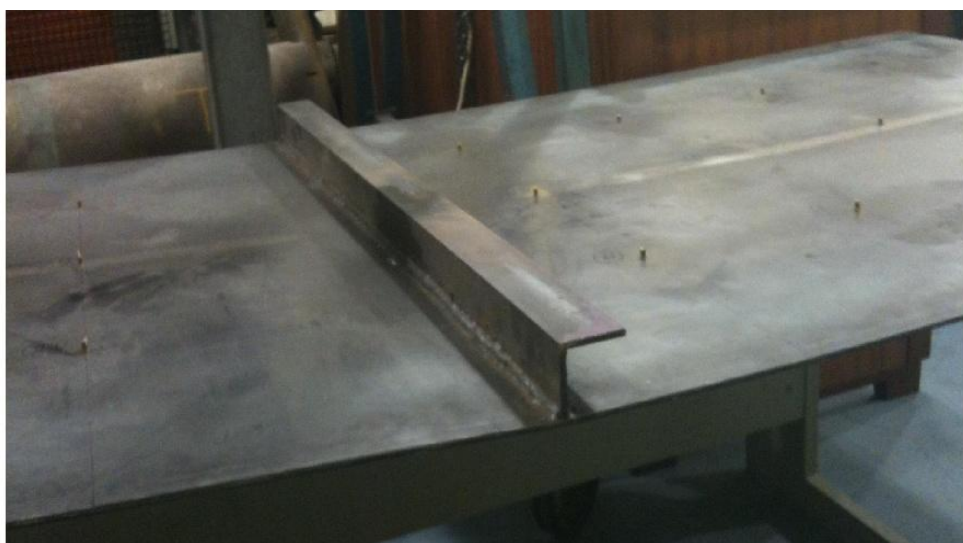
Fig 7.8 Stiffener of L-shaped cross-section (50 mm x 50 mm, 5 mm thick) welded on steel plate (size: 2 m x 1 m, 5 mm thickness).
