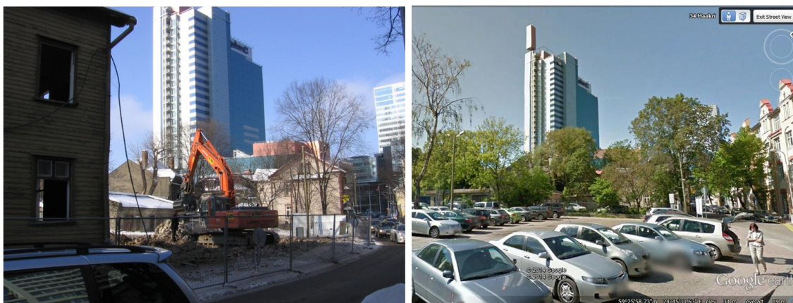
Figure 7.1. The development of a parking lot site. Photo on the left depicts demolition of old buildings (Source: Author's photo from 2006) and photo on the right is a today's parking lot (Source: Google Earth)
