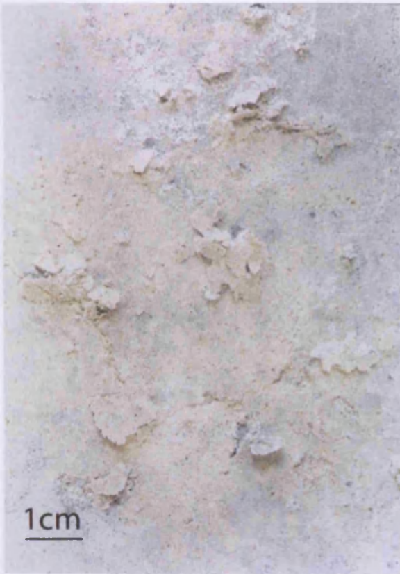
Figure 15 Salt crust and lime wash flaking in MD
