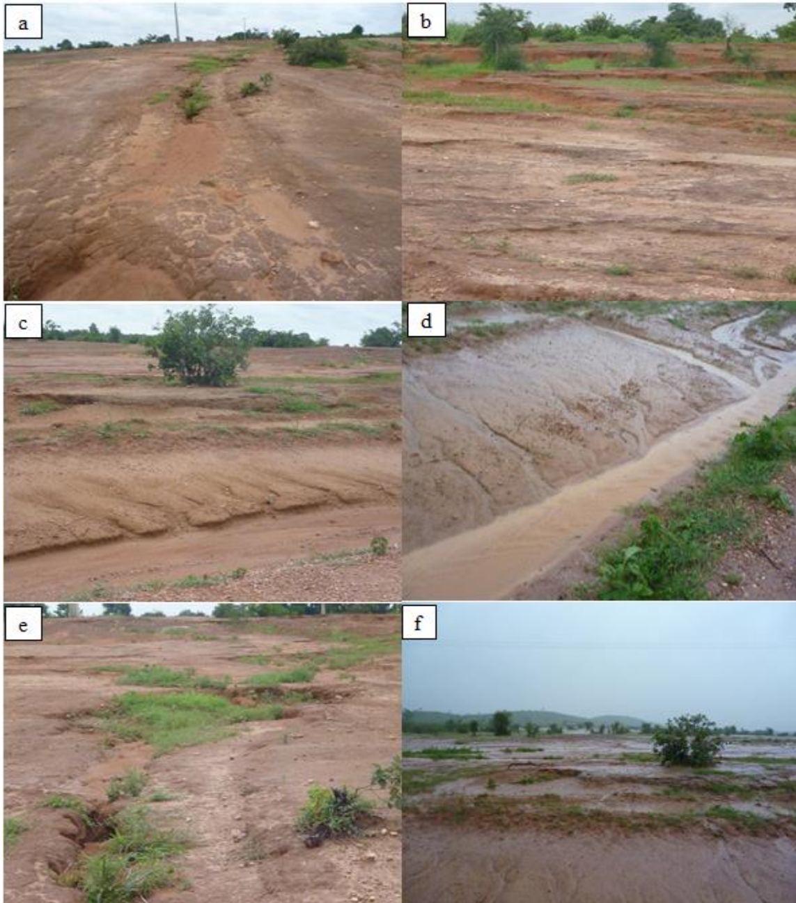
Figure 4.7: Pictures showing the (a-b) Crusted/Sealed layer and lack of vegetation during the rainy season; (c-d) Runoff channels before and during rainfall showing evidence of erosion; (e-f) eroded gullies in the sealed layer providing avenue for small vegetation growth /surface stripping
