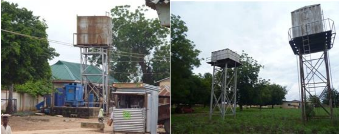
Figure 2.9: Non-functional mechanized pump boreholes with elevated tanks
