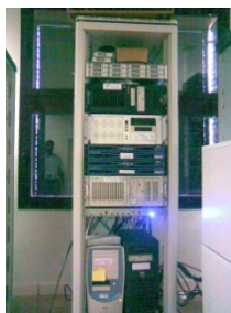
Figure 1. Photograph of the servers’ room
