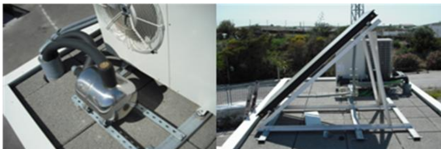
Fig. 4-7: HVAC equipment on the roof [DRA-SEIS]
