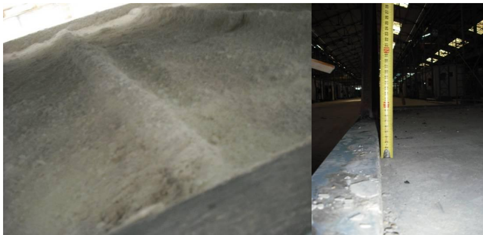
Fig. 4-6: Details of the floor slab: mineral wool mortar and space for the installation of the UFH system [DRA-SEIS]
