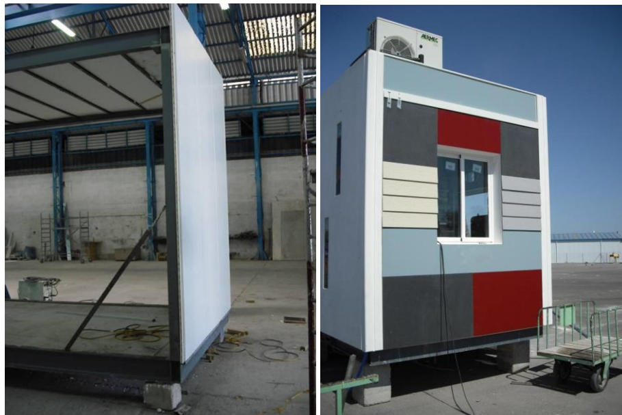
Fig. 4-22: Left, façade P-06 featuring the sheet-metal panel before being clad with composite panels; Right, P-12 featuring different finishing sideboards [DRA-SEIS]
