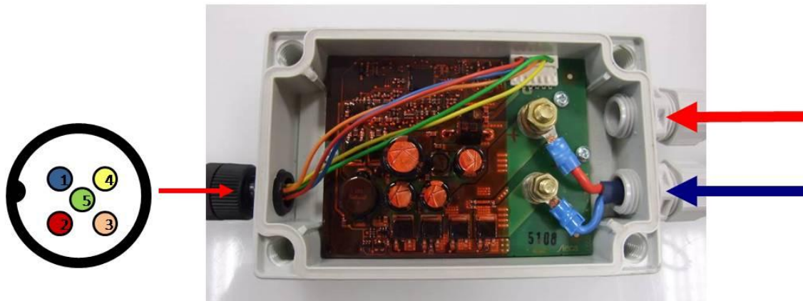
Fig. 4-31: ECGU Control box with the pin connector (left side) and the voltage (red) and ground (blue) cables [SGR]
