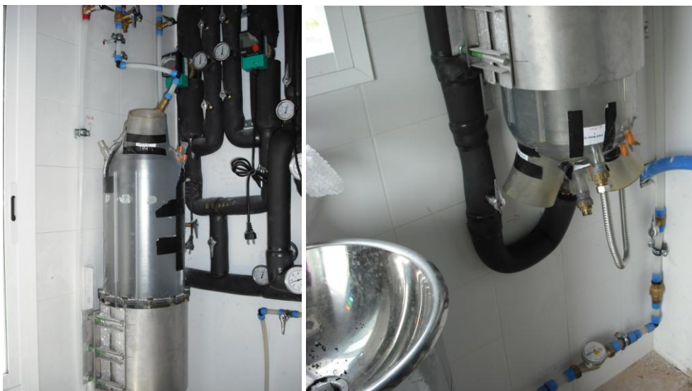
Fig. 4-33: MSTS fitted in the Mock-up kitchen: it can be seen the inlet and outlet runs, the water bypass and the operational sink [DRA]
