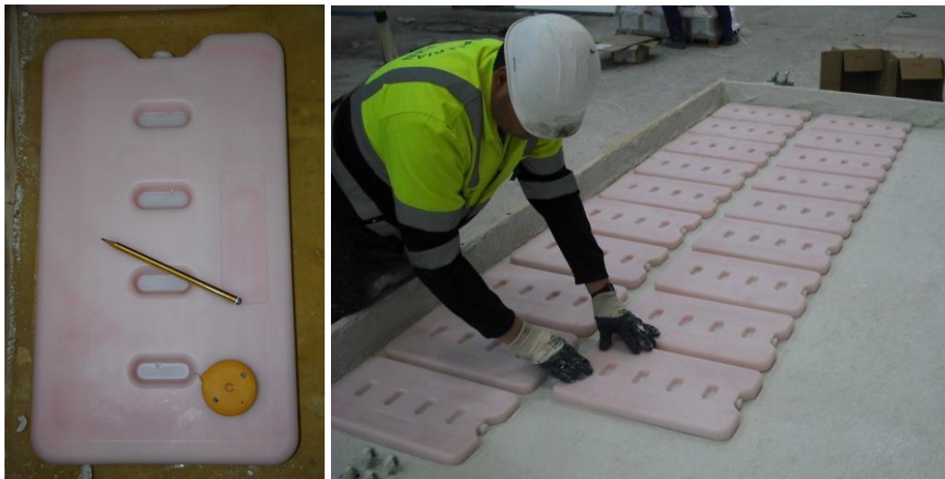
Fig. 4-10: PCM boxes and installation within the core of the sandwich panel by specialized factory staff, over the innermost GRC skin [DRA-SEIS]
