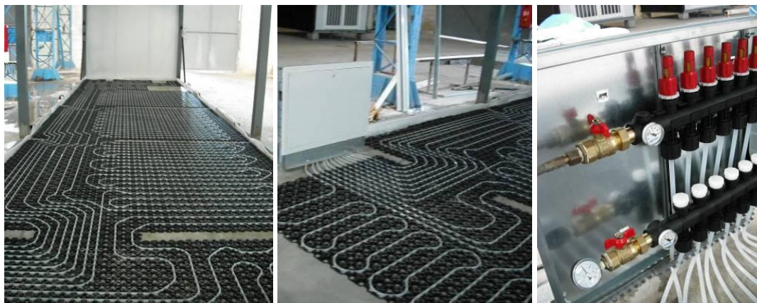
Fig. 4-26: UFH installation (left); all the circuits are collected in a manifold case (centre); water temperature and flow are controlled by the thermal drives (right) [DRA-SEIS]
