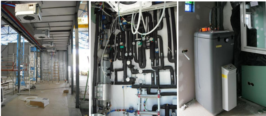
Fig. 4-32: Fan-coil units (left), pipes and controlling valves (centre) and water tank for DHW (right) [DRA-SEIS]
