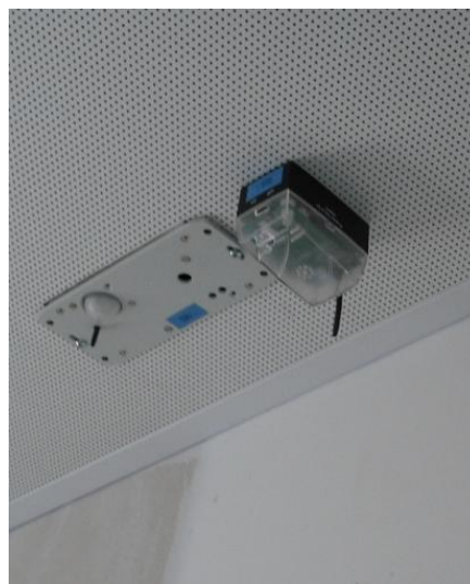
Fig. 4-36: C&P and HLT wireless sensors fitted in the Mock-up technical ceiling [DRA-SEIS]
