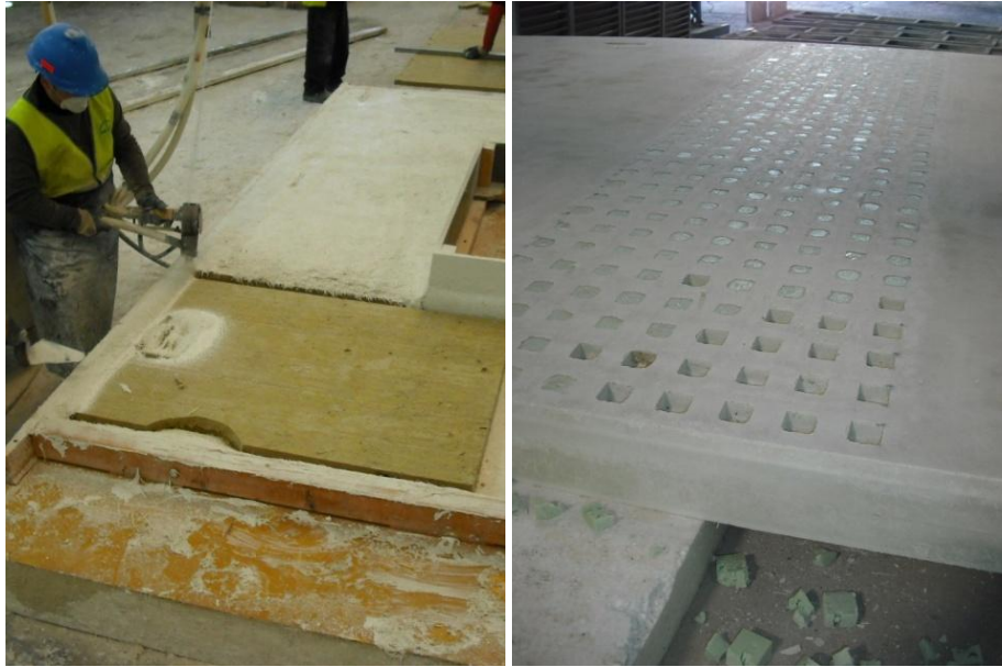
Fig. 4-21: Left, manufacturing process of the GRC sandwich panel with mineral wool filling; Right, special indoor finishing pattern for improving acoustical performance [DRA-SEIS]
