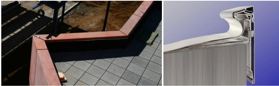
Fig. 2-5: Left, parapets at the CEDER building roof coping [DRA-SEIS]; Right, profiled aluminium drip guard with flexible waterproofing layer [Alwitra]
