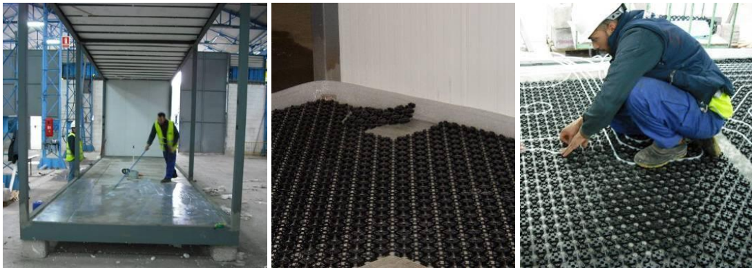
Fig. 4-25: Primer coating (left) and plastic chambers (centre) laid onto the Mock-up floor for the Mini UFH system water pipes, installed by specialist staff (right) [DRA-SEIS]
