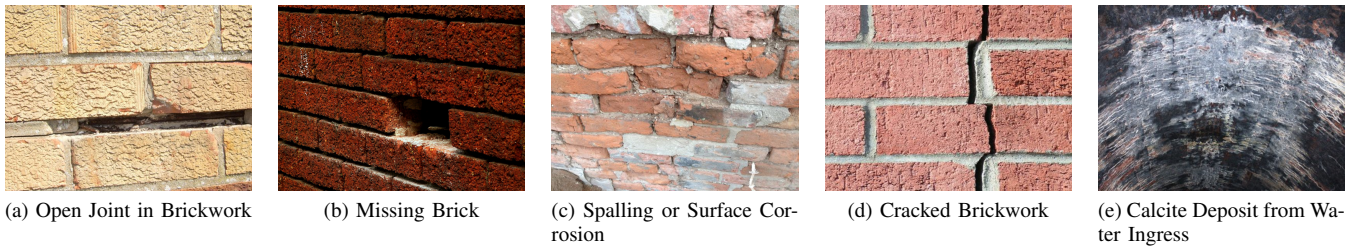
Fig. 1. Examples of various defects which examiners look for when conducting an inspection
