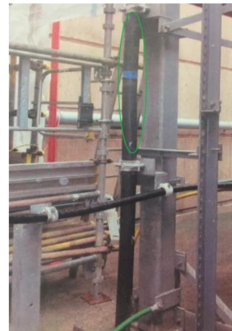
Figure 3. 275kV OF cable (Blue Phase) – the area marked in the green ellipse was observed to have a 5.2°C temperature rise.
