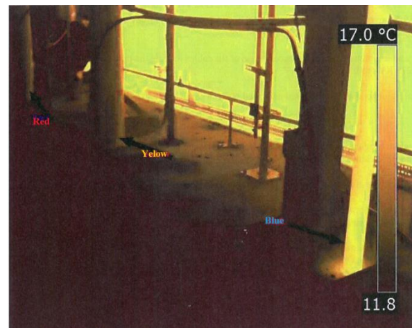
Figure 4. Infrared thermal image of the Blue Phase.
