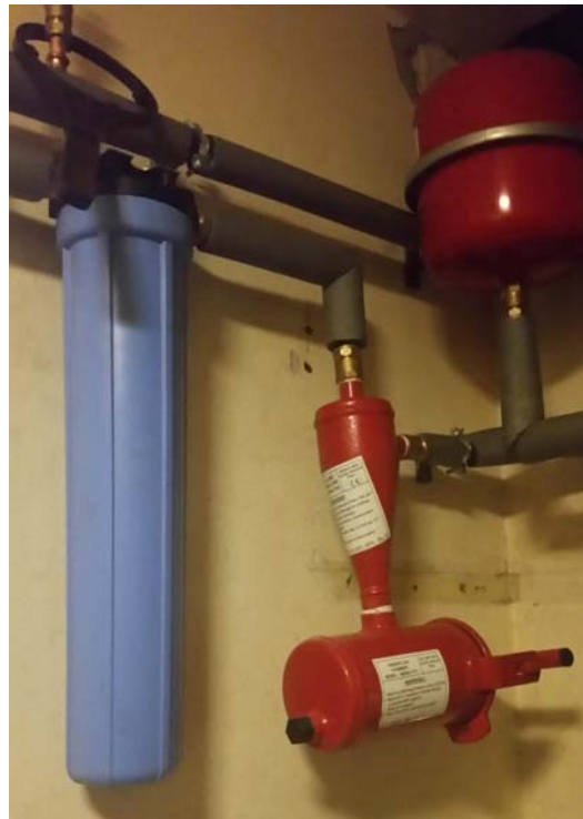
Figure 9: The water filter at the plant room
