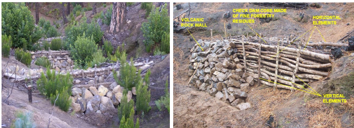
Figure 3 a) Series of mixed check dam colonised by the indigenous vegetation b) Elements of a mixed check dam
