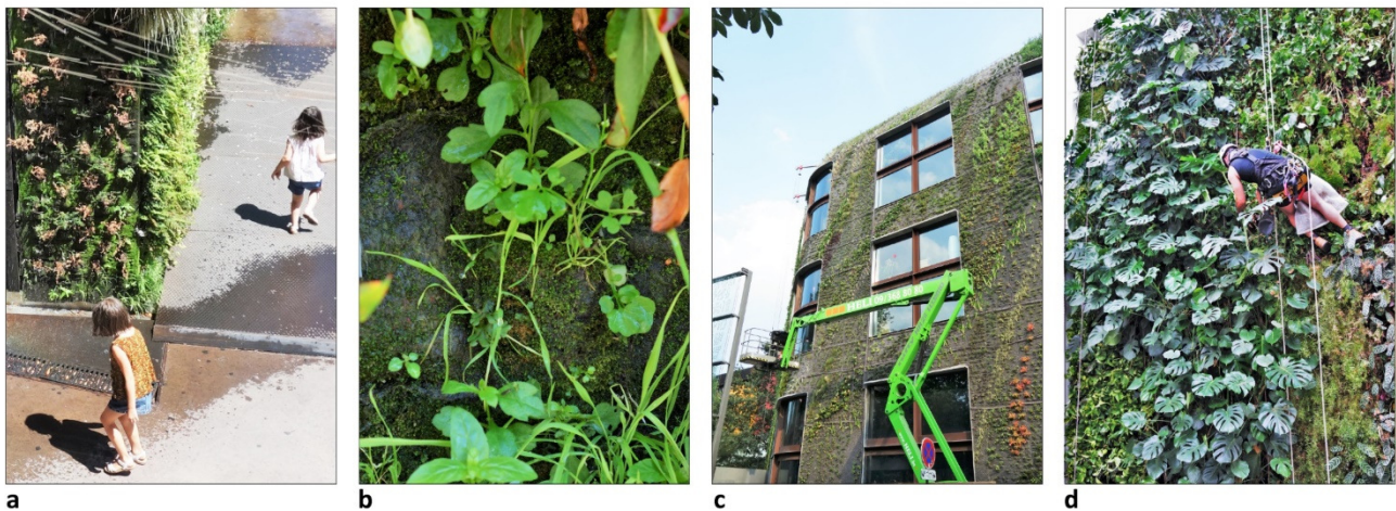
Fig. 6. Watering wastage (a); weeds taken root (b); replanting with articulated lift (c); canopy trimming by an abseiler (d).
