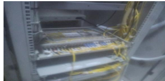
Gambar 2. Optical termination Box (OTB) (Sumber : PT. Telkom Pontianak)
