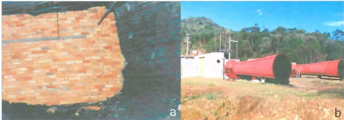
Figura 3.6 Tapumes de alvenaria (a) e exaustor principal (b).
