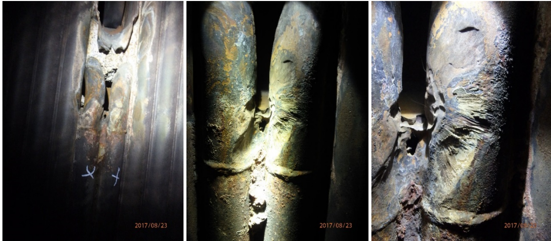
Figure 12. Corrosion below the urea injection lances.
