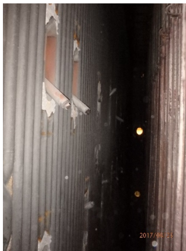
Figure 3. Commercial urea injection lances on the boiler front wall; secondary superheater on the right.
