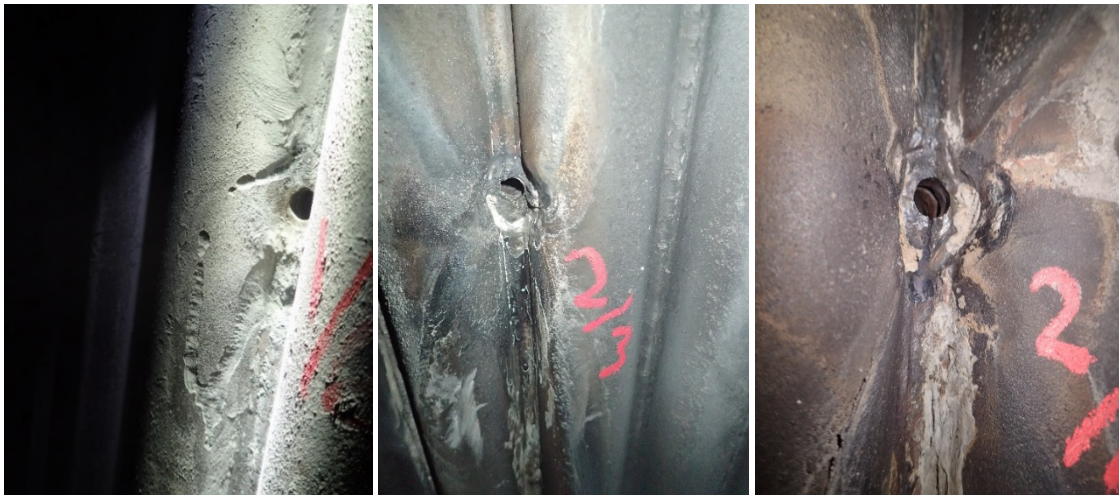
Figure 4. Corroded holes for injection nozzles inside the boiler.
