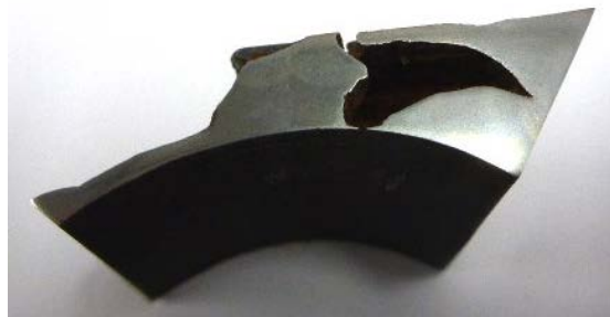
Figure 6. A corroded tube sectioned for microscopic examination; fireside on left, place for injection nozzle on top.
