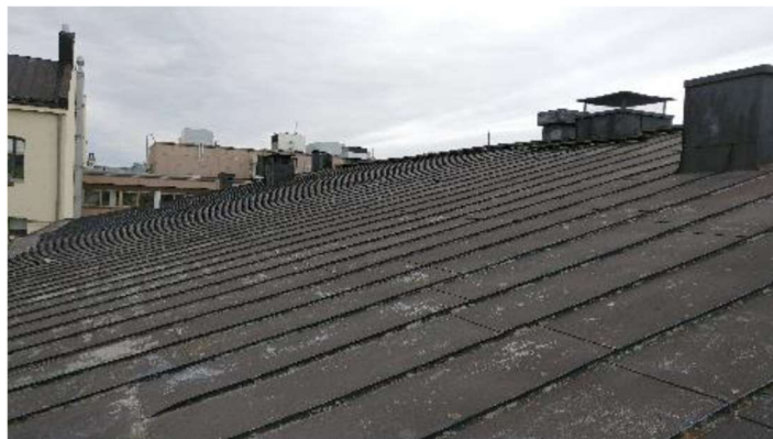
Figure 6. Tar felt containing PAHs. Photo: Jarno Komulainen, Vahanen Building Physics Ltd
