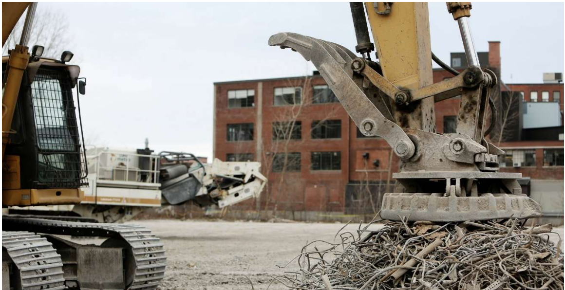
Figure 12. Electromagnetic lifting of steel scrap.
