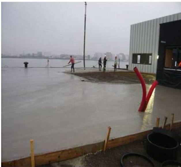
Figure 8. Ready-mixed concrete produced with 30% replacement of the coarse aggregates with recycled concrete aggregates 26 .
