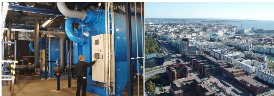
Figure 17: Installations in Helsinki
